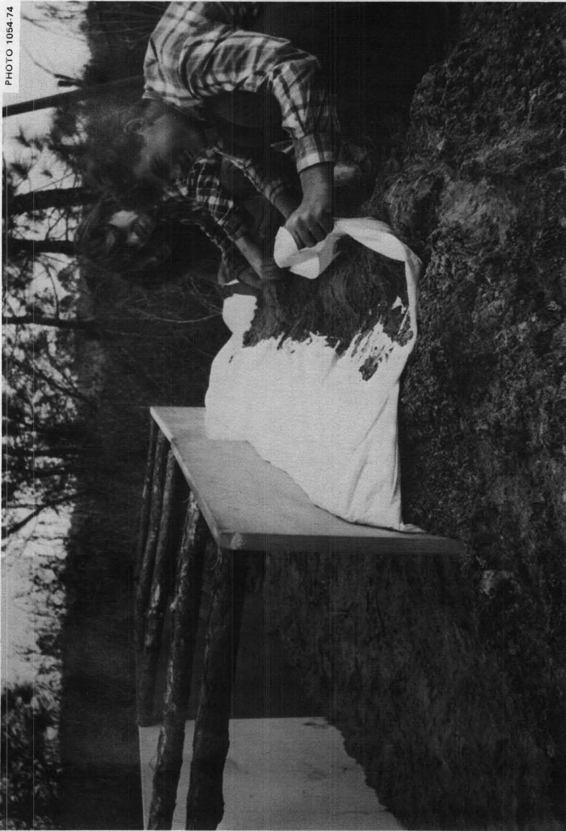
Fig. 5.58. Workmen building the first prototype of a shelter with vertical interior walls consisting of 2 or 3 rolls, stacked one on top of the other. This photo shows the workers forming an earth-filled "hook," which holds the part of a sheet forming the upper side of a roll in place, so that especially the vertical inner side of the roll will remain in place when the door form is removed.
